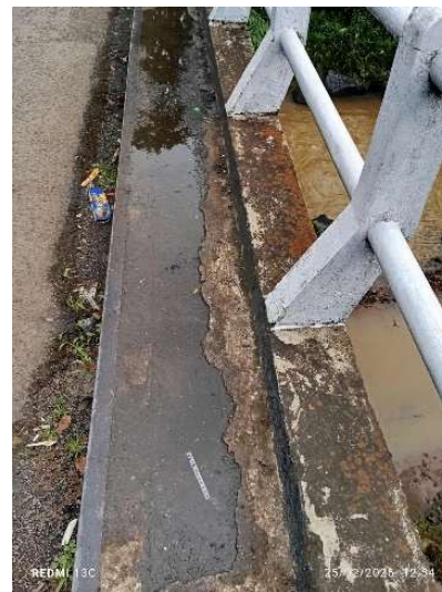
Figure 4 Malfunctioning bridge drainage system
