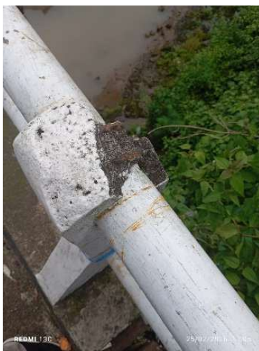
Figure 6 Damage on bridge railing elements
