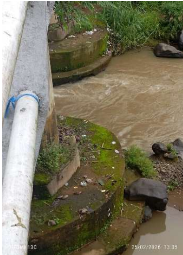
Figure 5 Scouring around the bridge pier area
