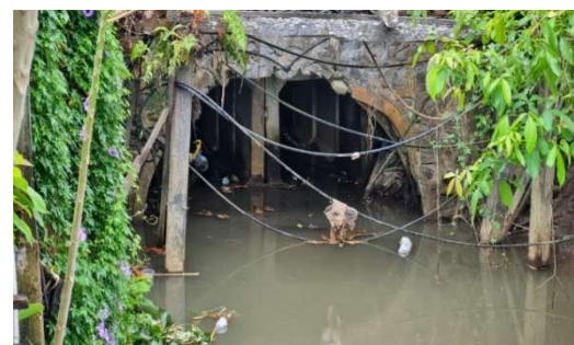
Figure 3 Scour-induced erosion at arch element (A1)
