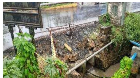
Figure 4 Arch failure due to settlement and slope instability
